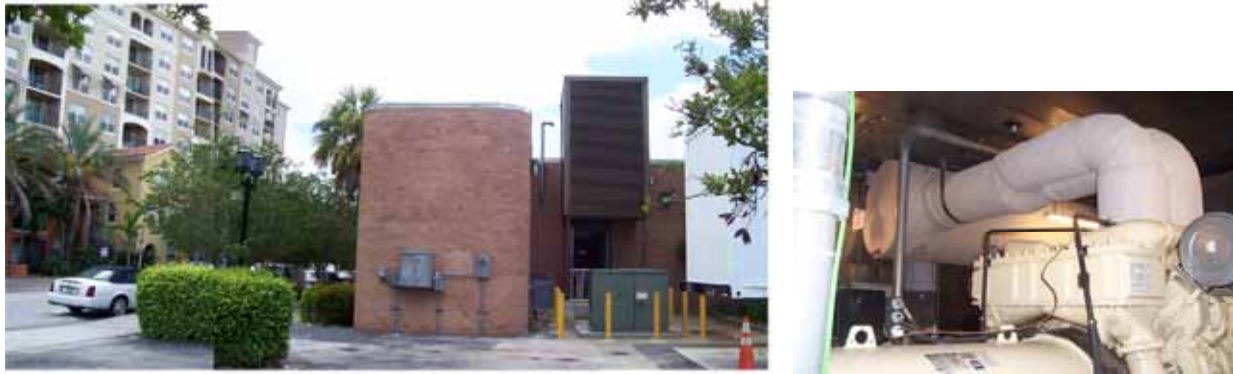
Figure 6: Some photographic images of the emergency generation plant building in proximity to the multi-level condominium building.
